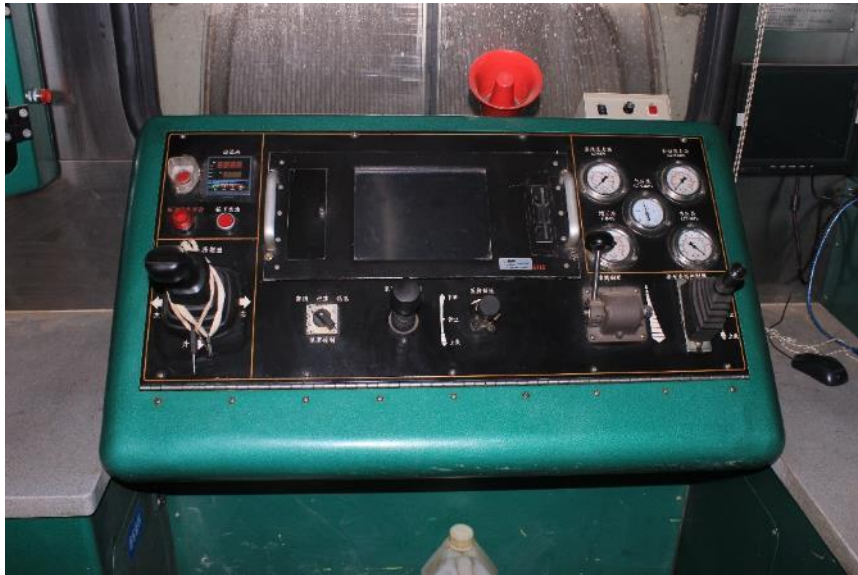
Figure 3-3 Drawworks console onsite
